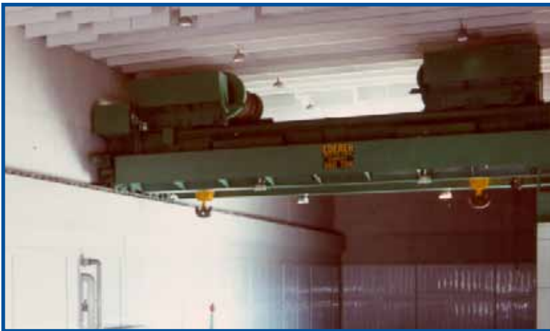
Turbine Building Crane
