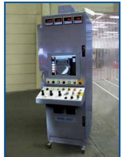
Modernized Control Panel
