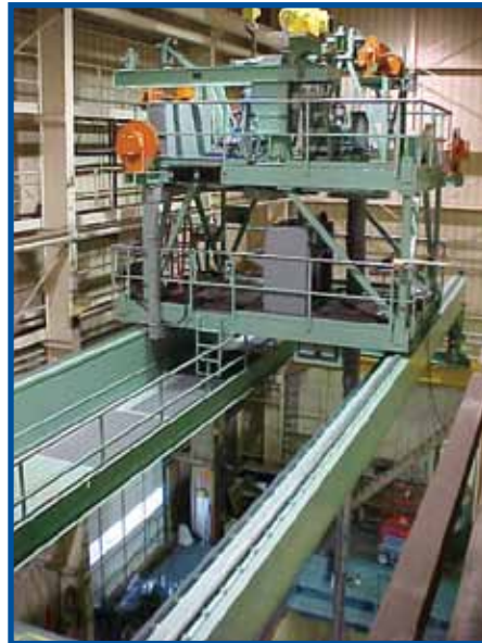
Refueling Platform (ABWR)
